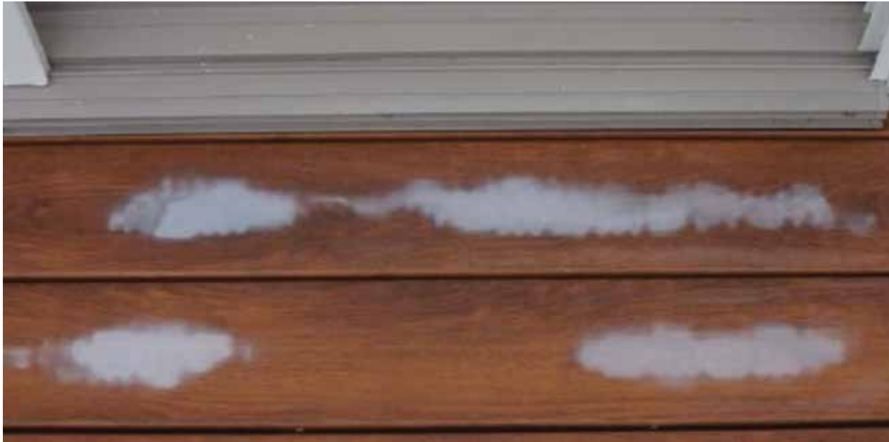
Example of discoloration that can be caused by using these products on Zuri Deck.
